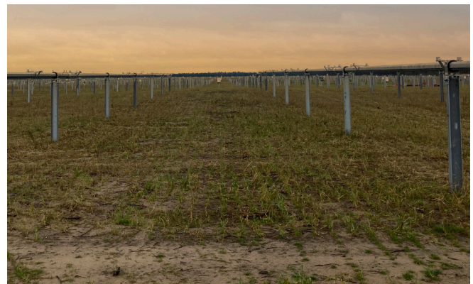
Piles and racking fully installed and await solar panels (Wood County Solar Project, Wood County, WI).
